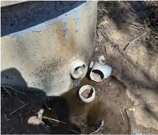
Septic pipe damaged in Blue Mtn Park
