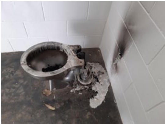
CWA Amenities vandalism
