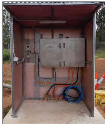
Figure 2: New electrical switchboard for Balance Tank
