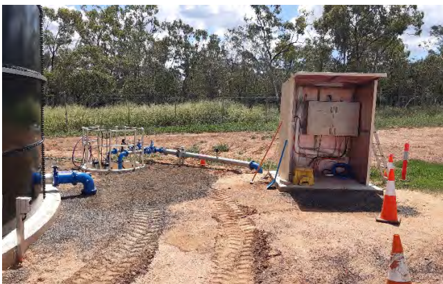
Figure 3: Pump well and switchboard shed
