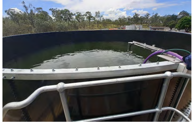
Figure 2: Balance tank full of recycled water during testing
