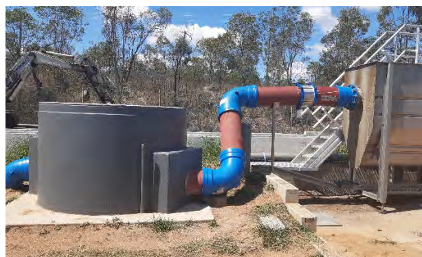
Figure 6: Wearer box and associated pipework (diverts the raw sewage to the balance tank).
