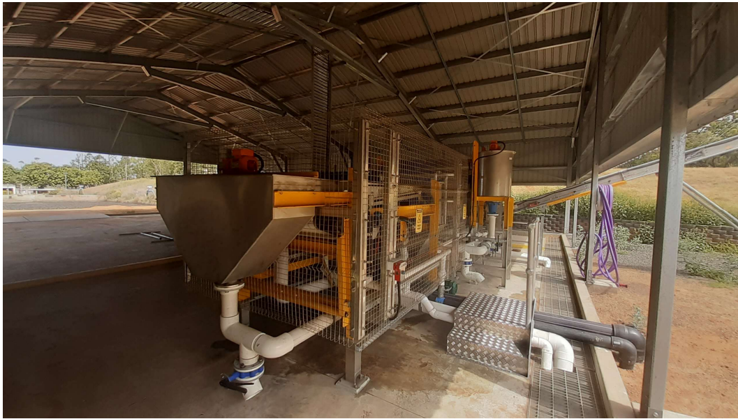
Figure 2 – Moranbah BFP – Final installation
