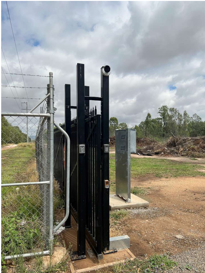
Automatic gate at Wowan Transfer Station
