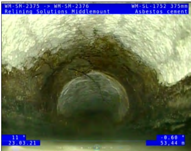
Figure 3 – Disintegrated 375 AC main MMT, section of pipe missing
