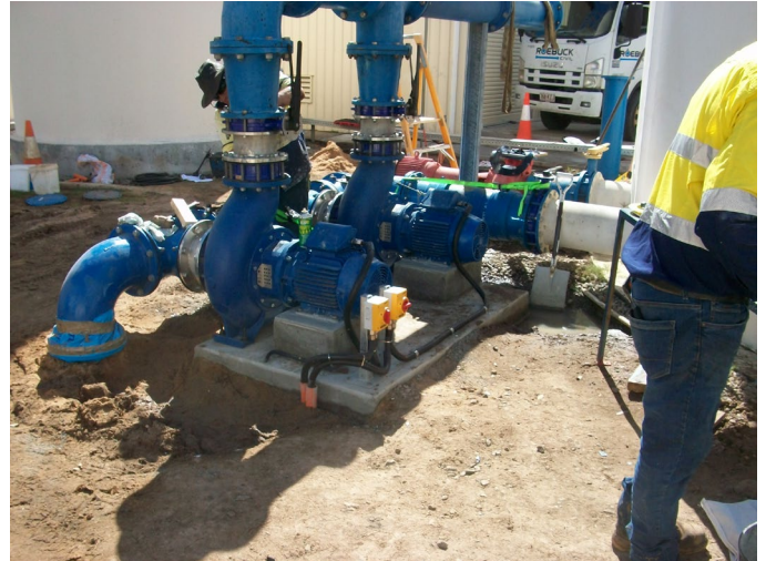
Figure 5 – New filter backwash pumps
