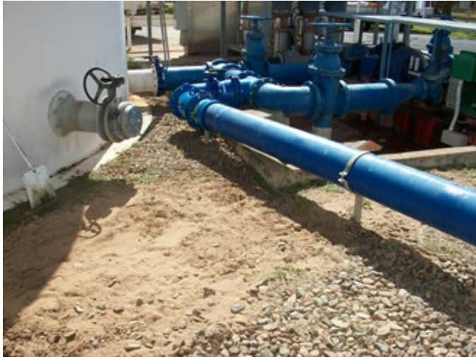
Figure 4 – New outlet pipework
