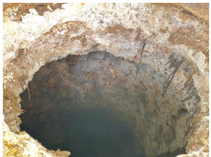
Figure 2 – Image of manhole attacked by hydrogen sulphide (H2S) gas in Middlemount
