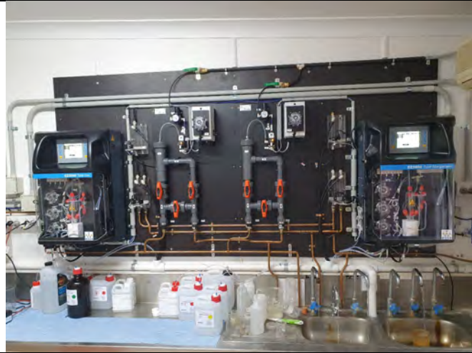
Figure 1 – Analysers in WTP lab room
