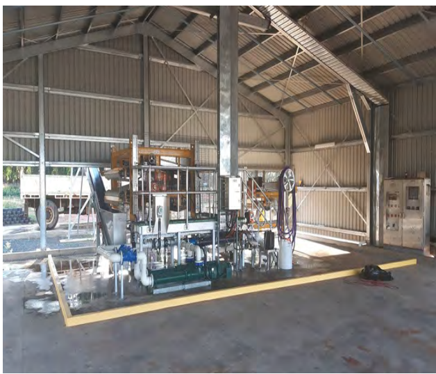
Figure 1 – Belt Filter Press setup
