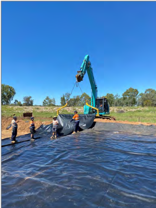
Figure 5: The installation of the liner for the storage area for the geo tubes
