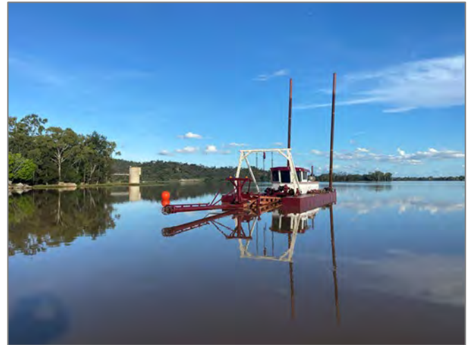
Figure 6: The barge being floated which will be stored in the exclusion zone beside the offtake tower
