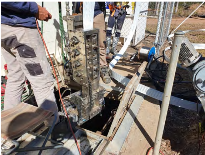
Figure 1 – Spiral winding machine installation at Middlemount PS #01
