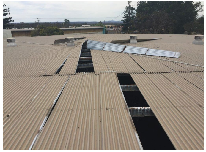
Figure 2 – Current roof condition displaying damage to roof sheeting
