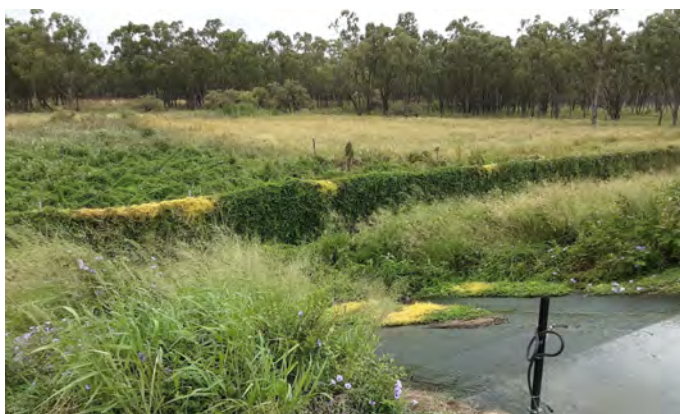
Moranbah Spillway Overtopping
