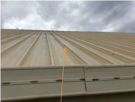
Dented roof sheets
