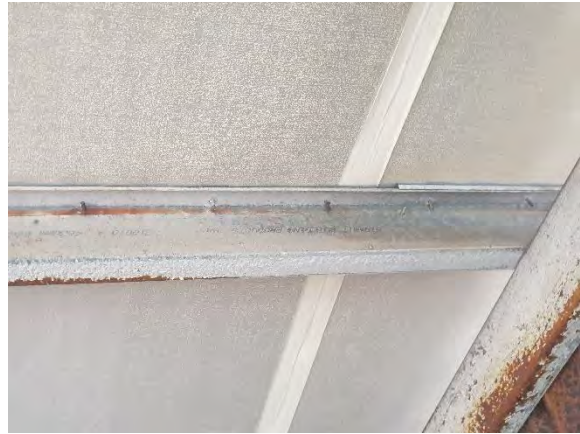
Rust to structural roof members
