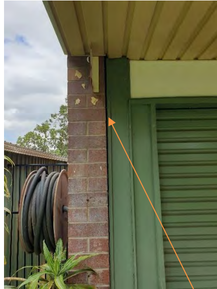
Brick wall separation from Storeroom
