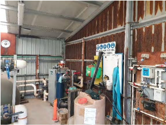
Rust to structural members and wall sheets
