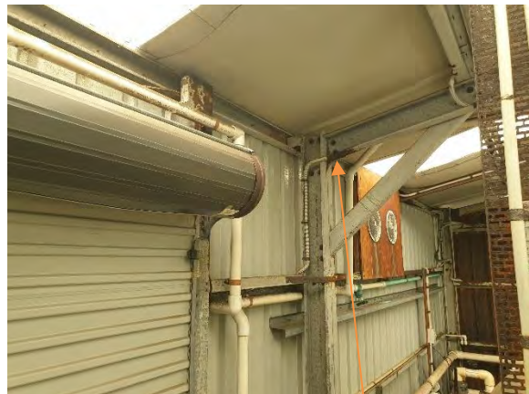
Rust to structural connections
