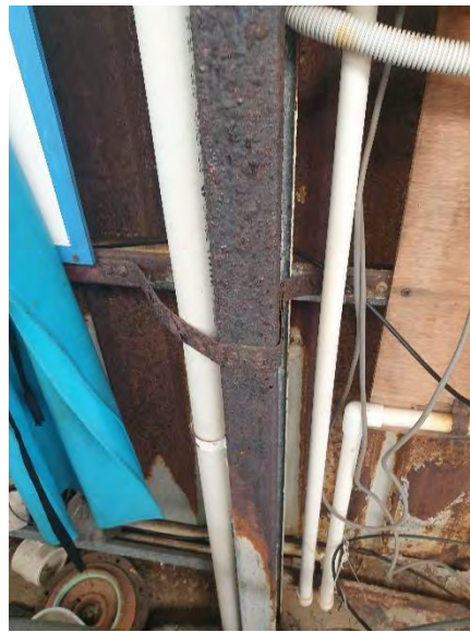
Rust to structural members and wall sheets
