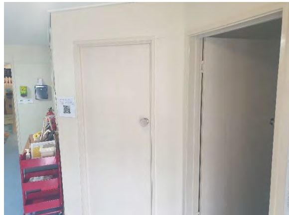
Cracking to wall lining
