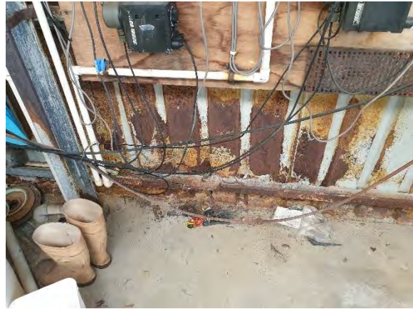
Rust to structural members and wall sheets
