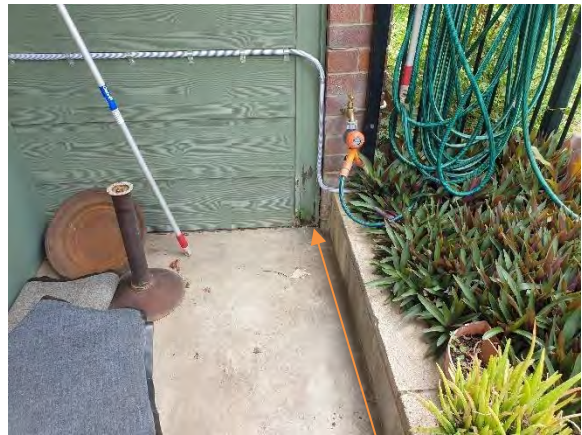
Rust at base of steel column
