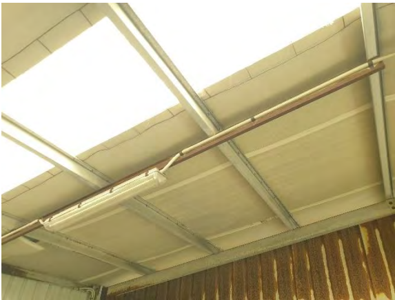
Rust to purlin bridging
