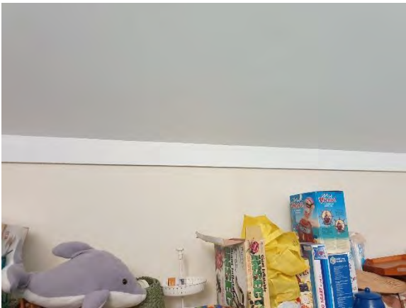
Water leak marks
