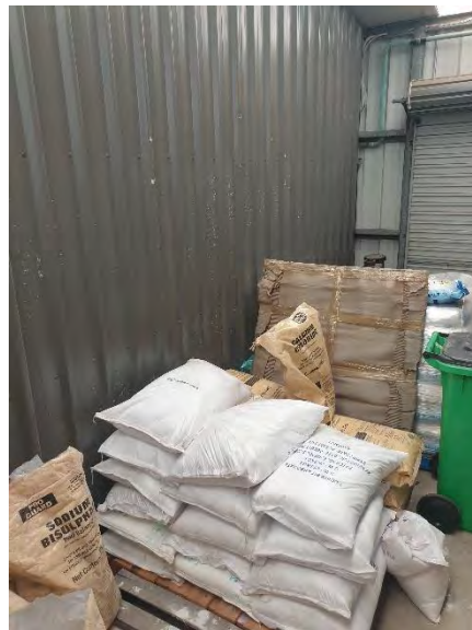
Rust to other side of wall sheets
