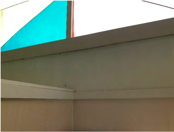
Water leak marks and damage
