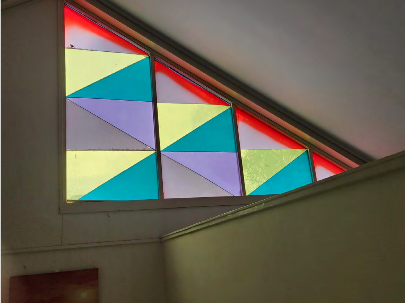
Figure 1 – North-facing perspex window with lifting of seals due to warping (bottom left corner).
