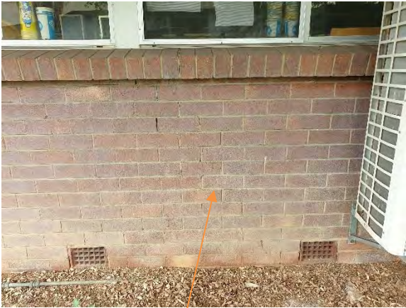
Minor brick cracking
