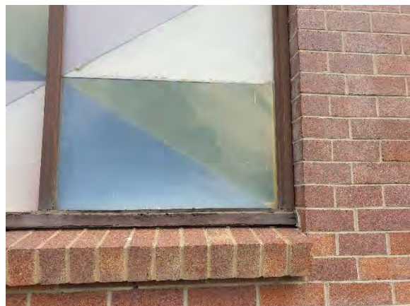
Windows and trims deteriorated
