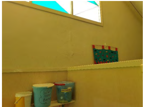
Water damage to wall lining
