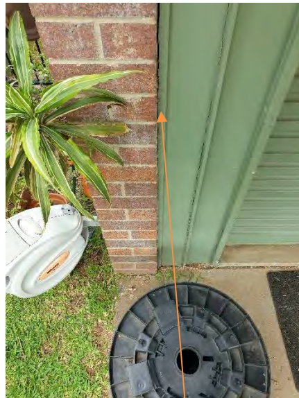
Brick wall separation from Storeroom
