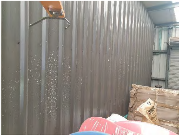
Rust to other side of wall sheets
