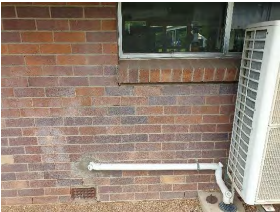
Minor brick cracking
