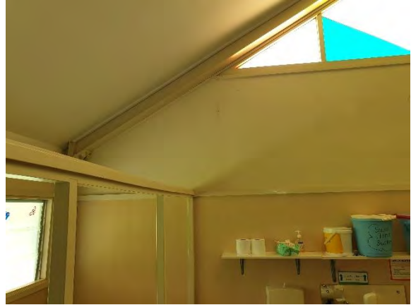
Water damage to wall lining
