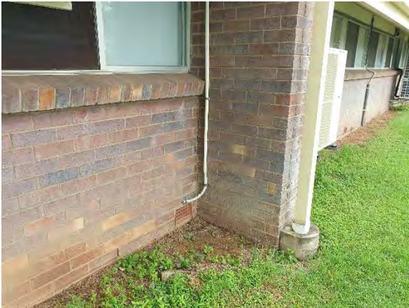
Minor brick cracking
