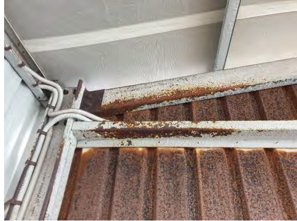
Rust to structural members and wall sheets
