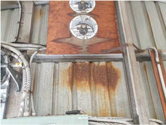
Rust to wall sheet below vents
