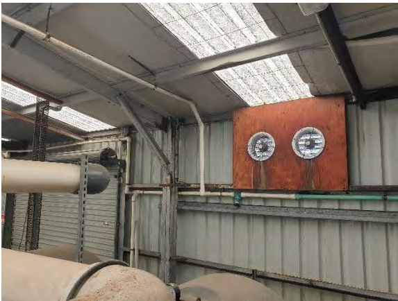
Rust to structural members and wall sheets
