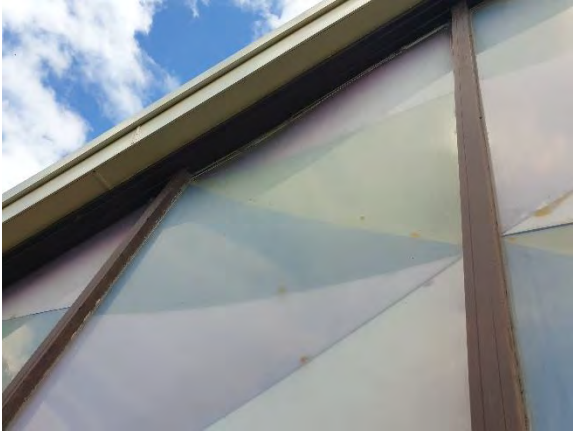
Windows and trims deteriorated.
