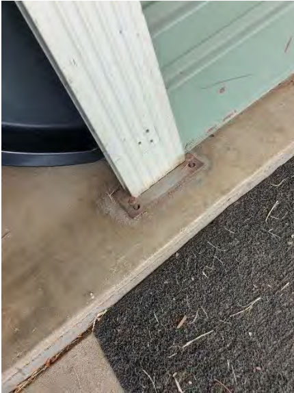
Roller door bolts not fastened
