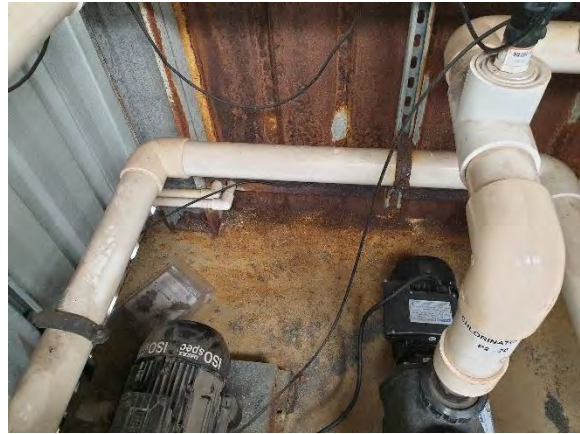
Rust to structural members and wall sheets
