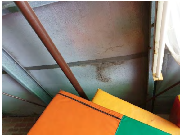
External storeroom water leak
