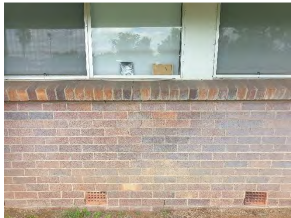
Minor brick cracking
