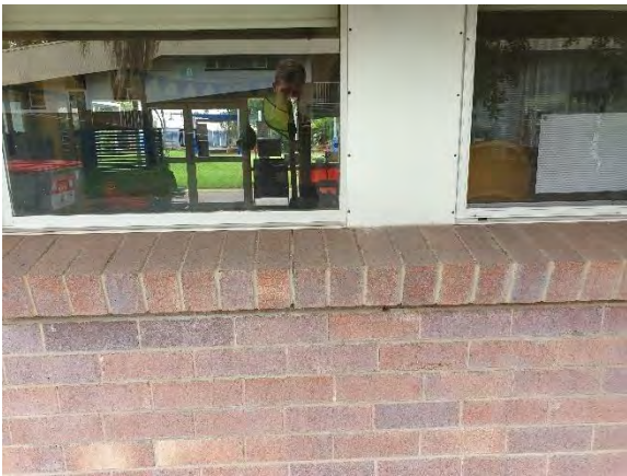
Minor brick cracking
