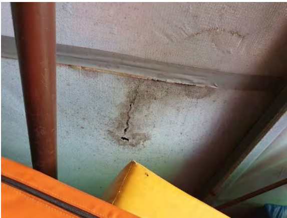
External storeroom water leak
