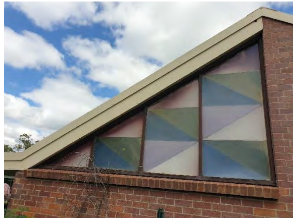
Windows and trims deteriorated
