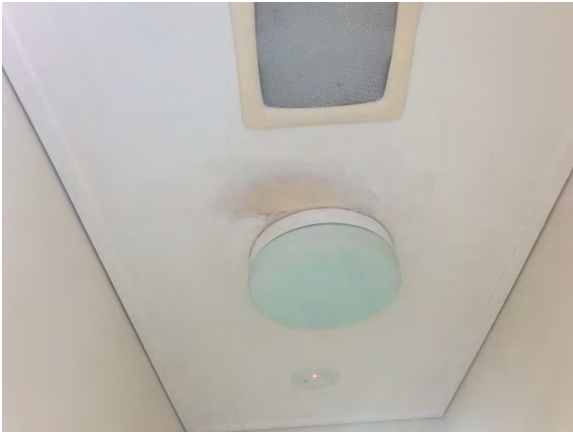
Roof leak in toilet
