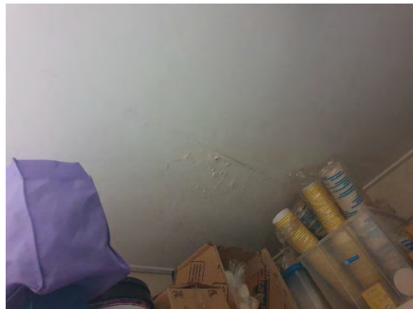
Roof Leak in Storeroom
