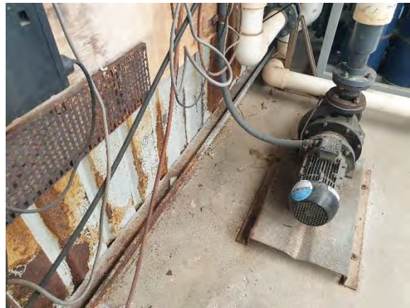
Rust to structural members and wall sheets
