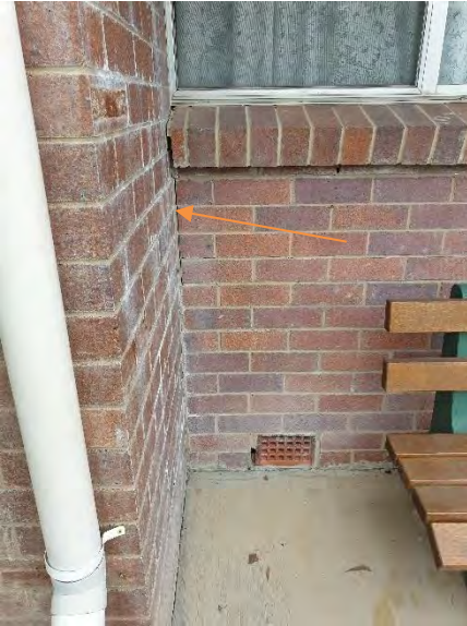
Minor brick cracking
