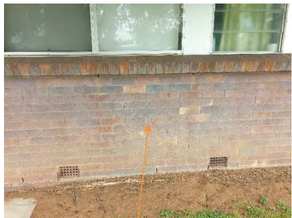
Minor brick cracking
