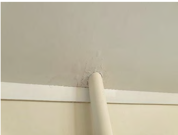
Water damage to vent pipe
