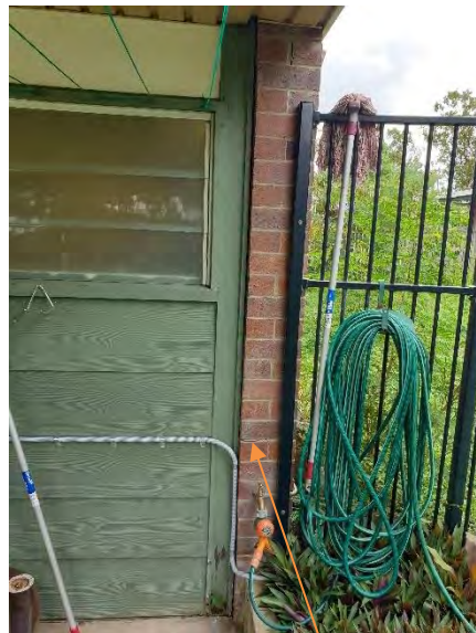
Minor brick cracking
