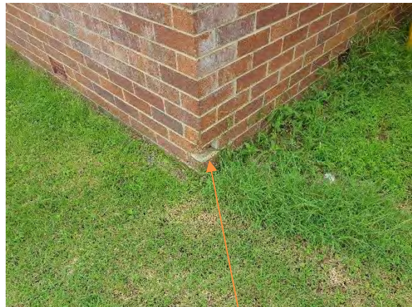
Brick damaged on corner
