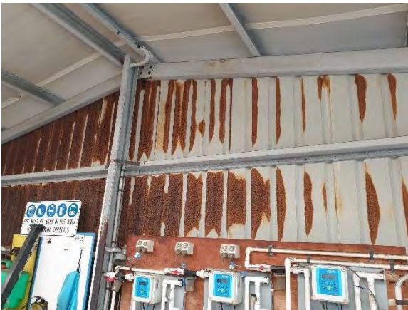
Rust to structural members and wall sheets
