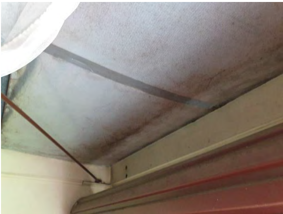
External storeroom water leak
