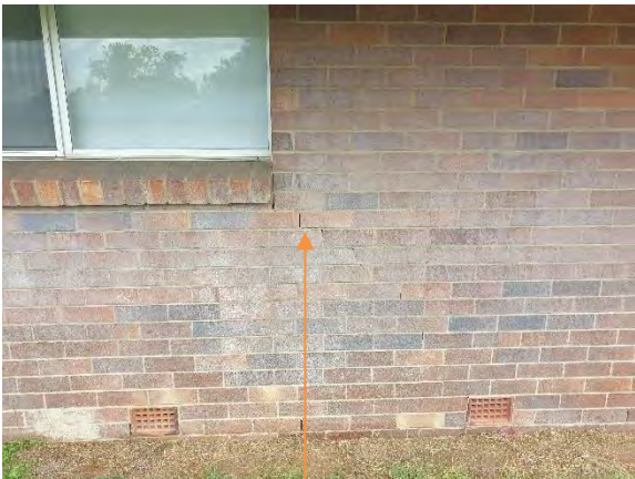
Minor brick cracking
