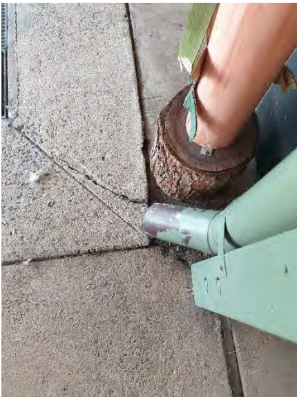
Slab movement affecting downpipe discharge
