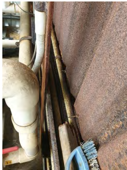
Rust to structural members and wall sheets
