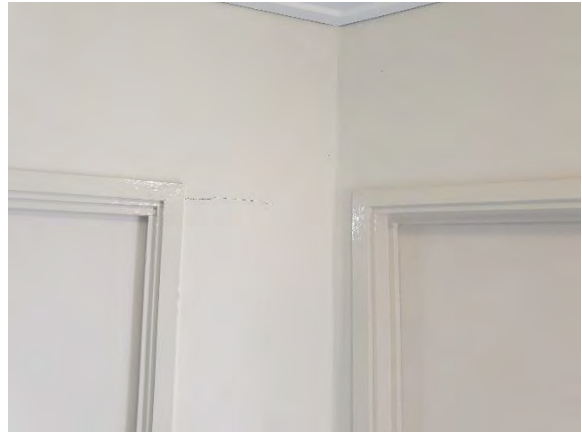
Cracking to wall lining
