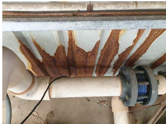
Rust to structural members and wall sheets
