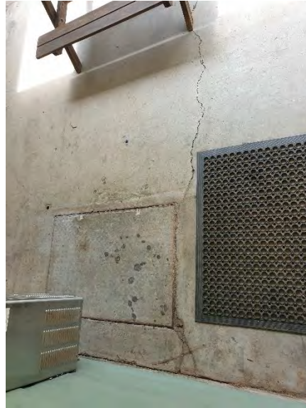
Concrete slab cracking
