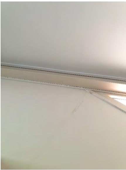
Water damage to wall lining
