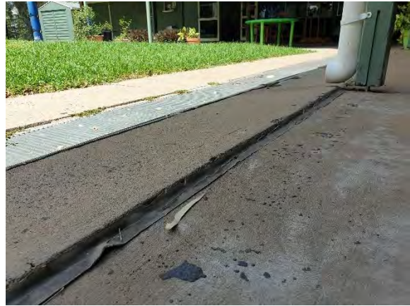
Sealant cracking and slab movement
