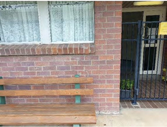
Minor brick cracking
