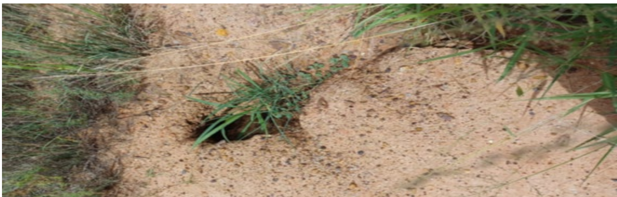
Moranbah ESD sinkhole before rehabilitation.
