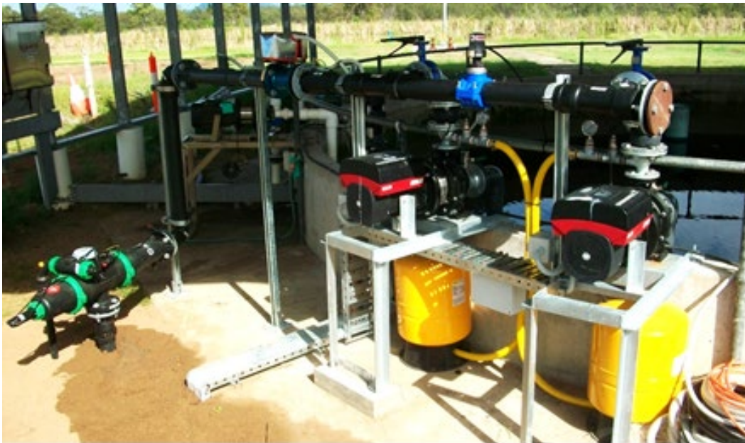
Photo 3 – Pump and filter assembly
