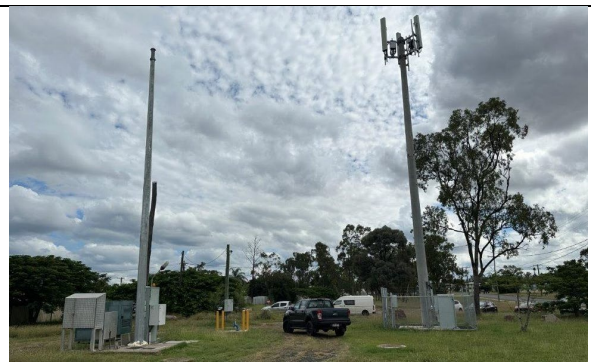
Photo 9 – SPDYS02 – 12m Vent pole
