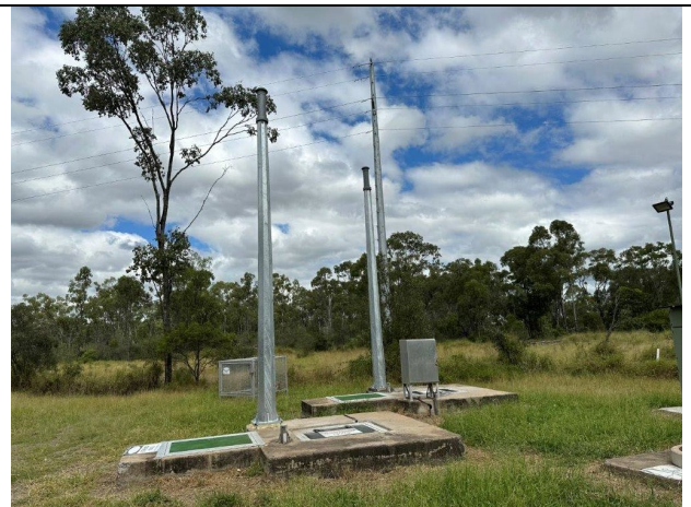
Photo 5 – SPMMT02 2x6m Vent poles and manhole covers
