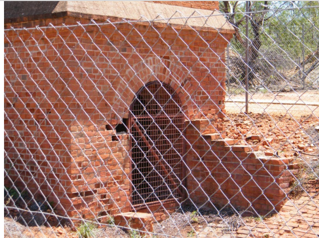
Base of the brick chimney stack showing safety mesh grill and current condition.
